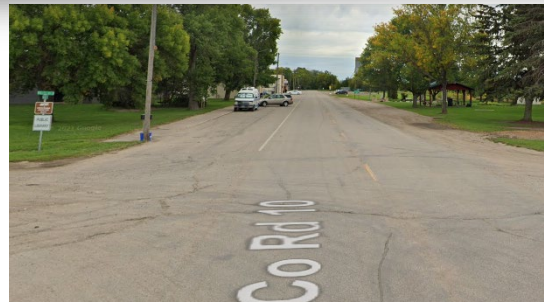
Road deterioration and lack of ADA accessibility
