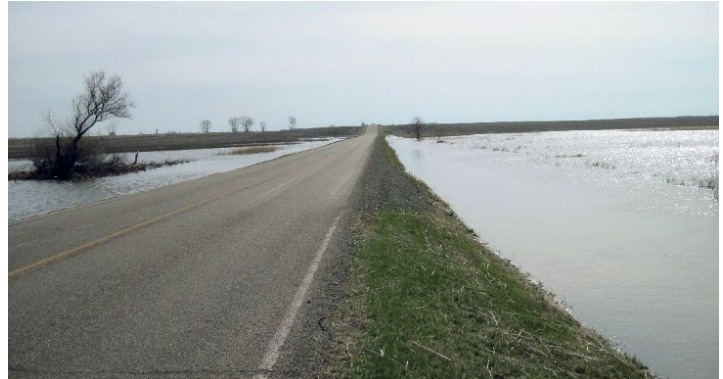
Lack of shoulder width and flooding from improper drainage
